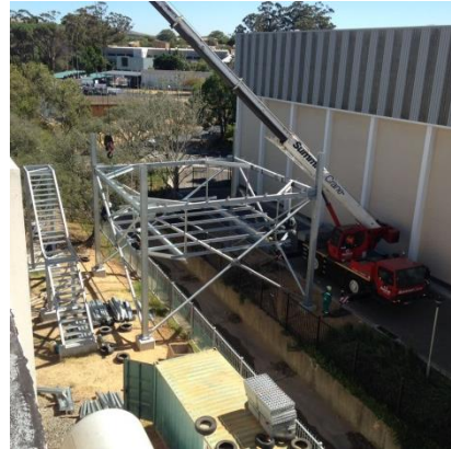
Erection of the Full Scale test facility at Stellenbosch University. © ENEXIO Germany GmbH & Kelvion Holding GmbH
