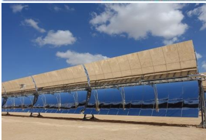
The parabolic trough power plant with collector area of 10,000 m 2 has an electrical power of one megawatt. © Fraunhofer ISE
